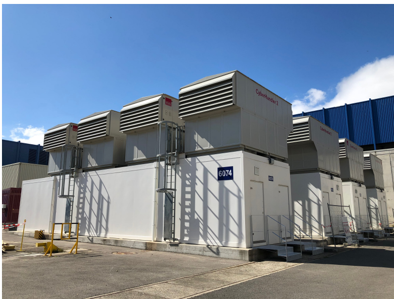
Figure 95. The ALICE CR0 data centre which houses the EPN farm.
