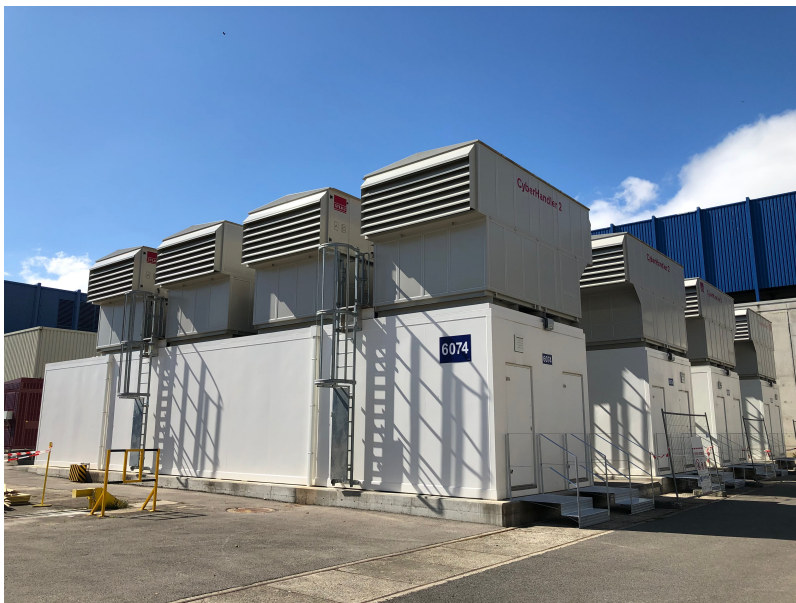
Figure 95. The ALICE CR0 data centre which houses the EPN farm.
