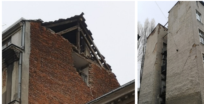
Figure 6. Photographs from damage assessment of the building after the Zagreb earthquake.
