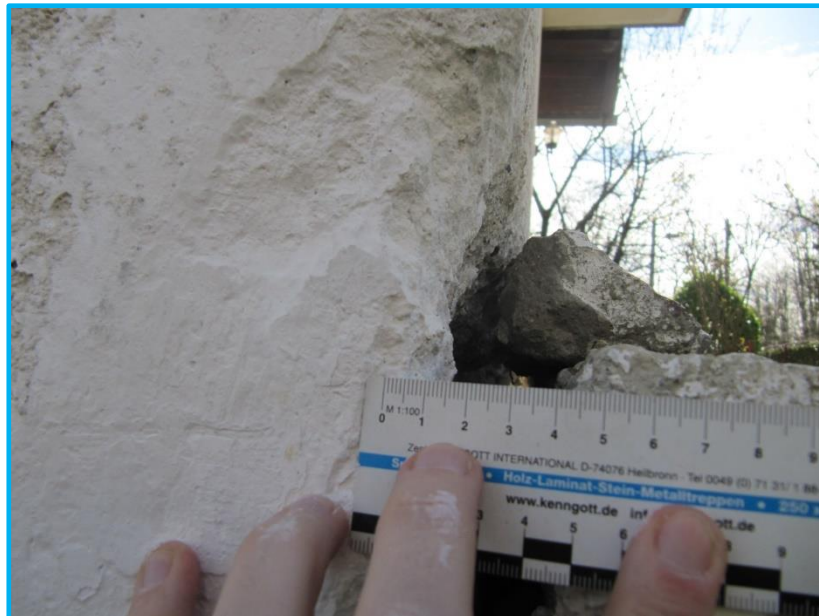
photo-244,245,11 → pukotina 5 cm
